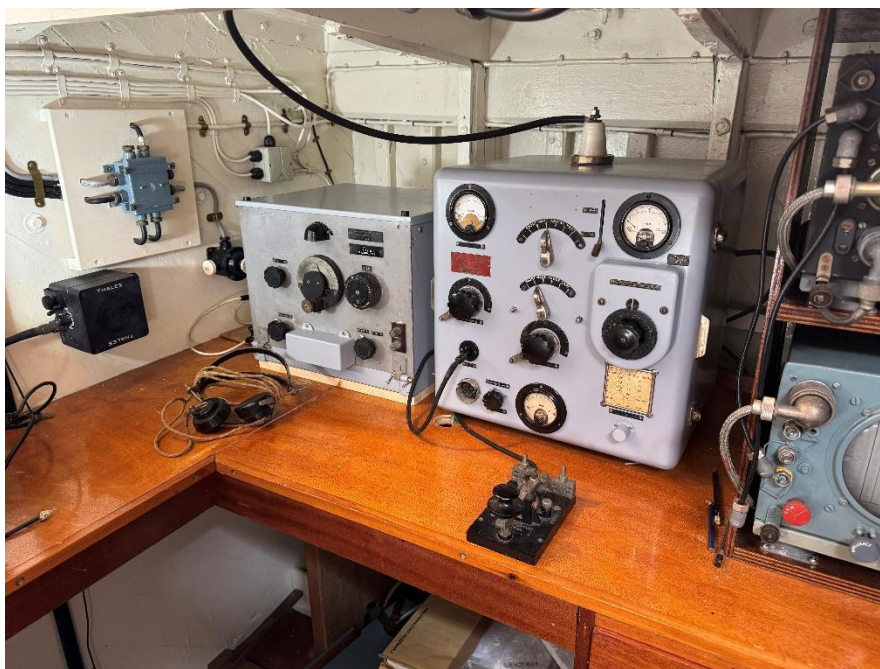
Marconi TW12 W/T installation.
